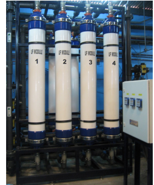
Figure 1. Ultrafiltration Modules of Kalinisan Wastewater
